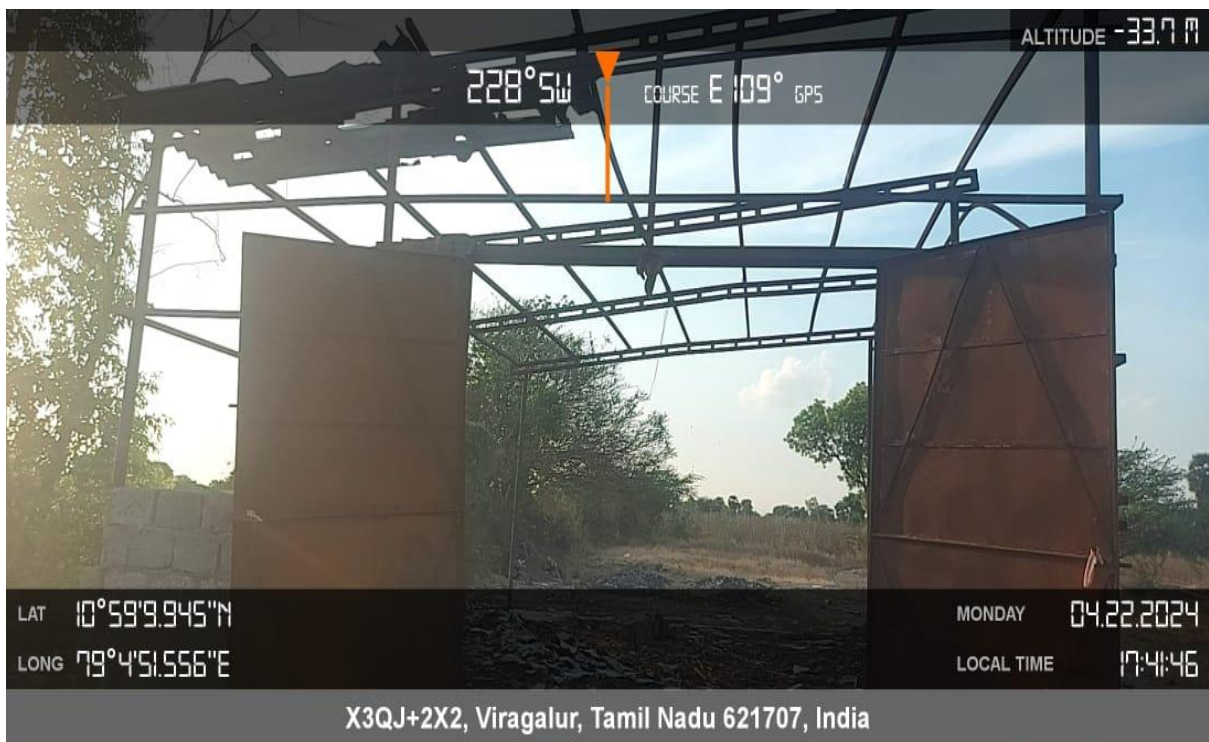
Steel structure of the damaged shed
